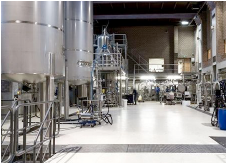
Bio Processing research plant
